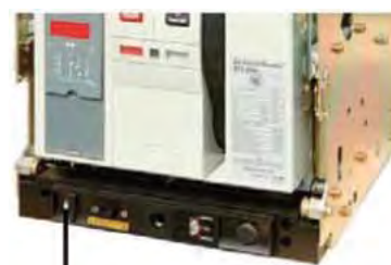
Safety padlock mechanism at the position of "separated"
