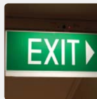
Emergency systems (emergency lights, security alarms, CCTV,...)
