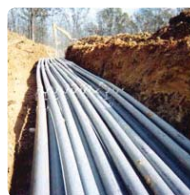
Connection to underground AC line
